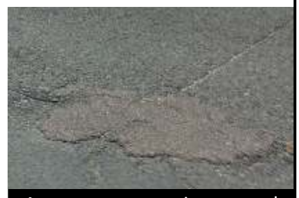
A temporary repair may only last a few months
